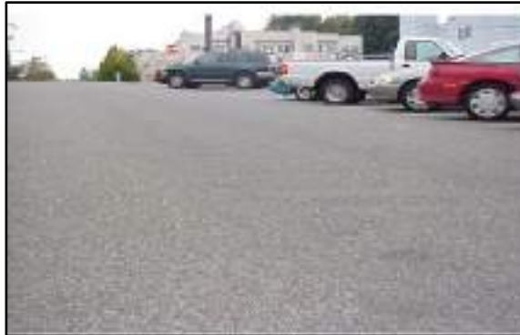
Gambar 2.10 Kerusakan Keriting ( Corrugation )
