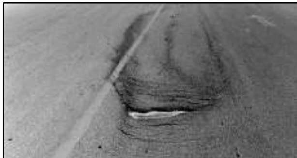
Gambar 2.5 Retak Bulan Sabit ( Slippage Crack )
